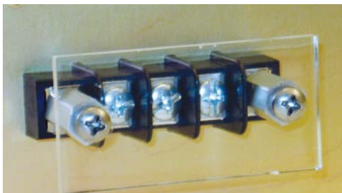
Installed Terminal Block front of Plate
